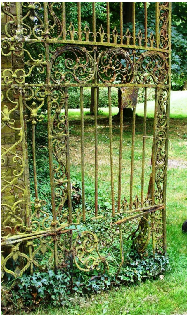
Picture 19. Fine entrance gates to Benington Lordship in urgent need of repair.
