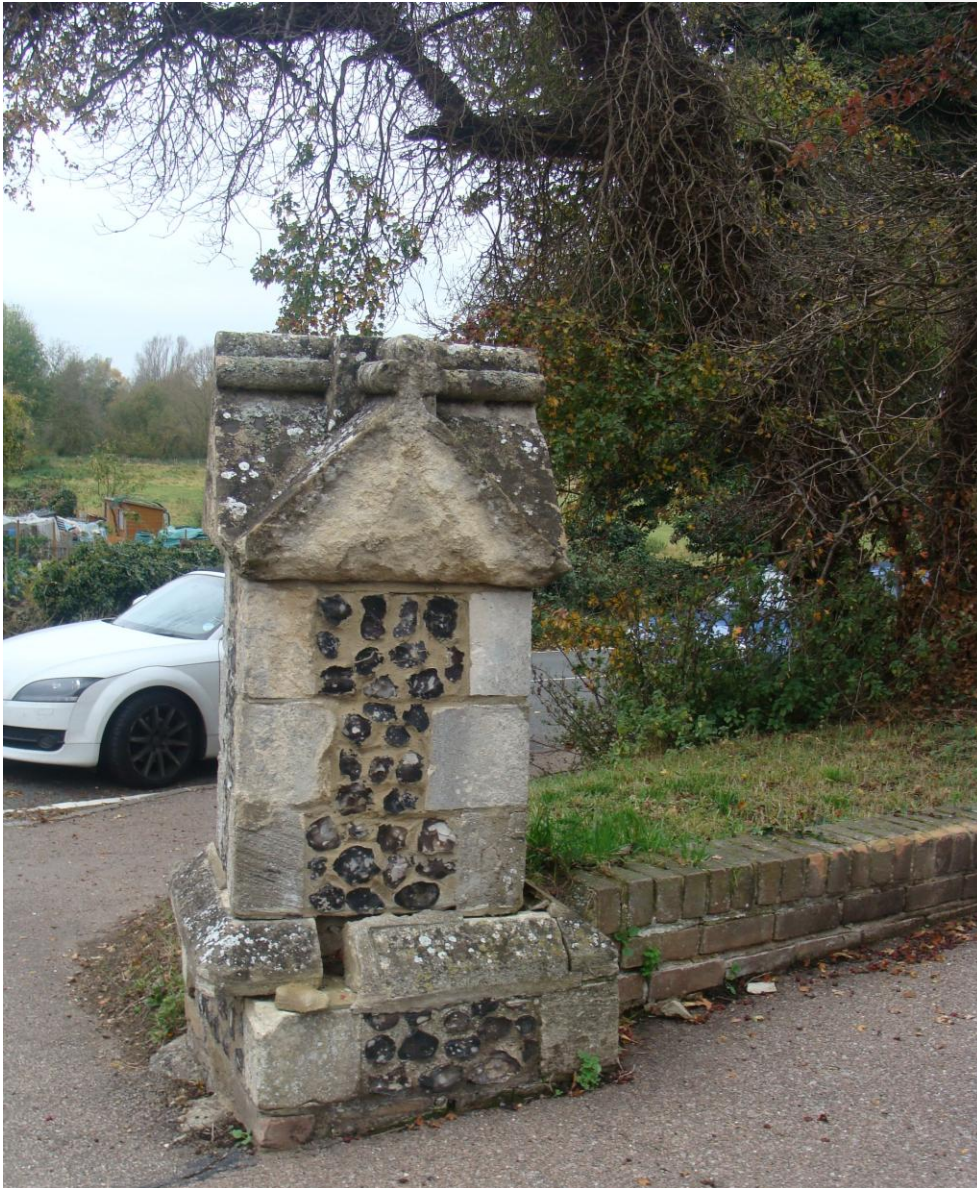
Picture 12 – Individually listed 19 th century grade II pier to St Andrews Church, Cappell Lane, in need of repair.
